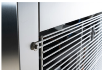
Anti-rodent grid at the back of the refrigeration unit.
